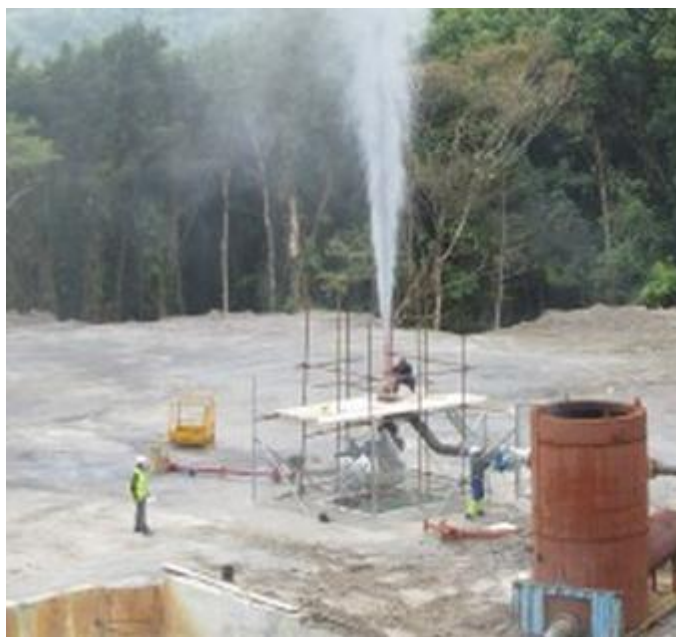
Geothermal well in Dominica
